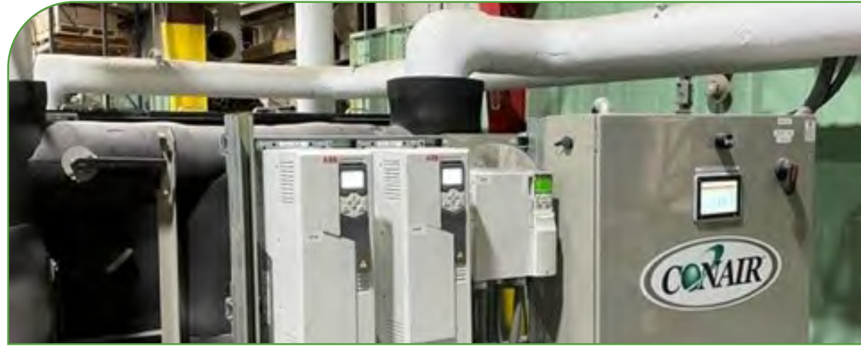
Closed-loop process water system in Biddeford, Maine
