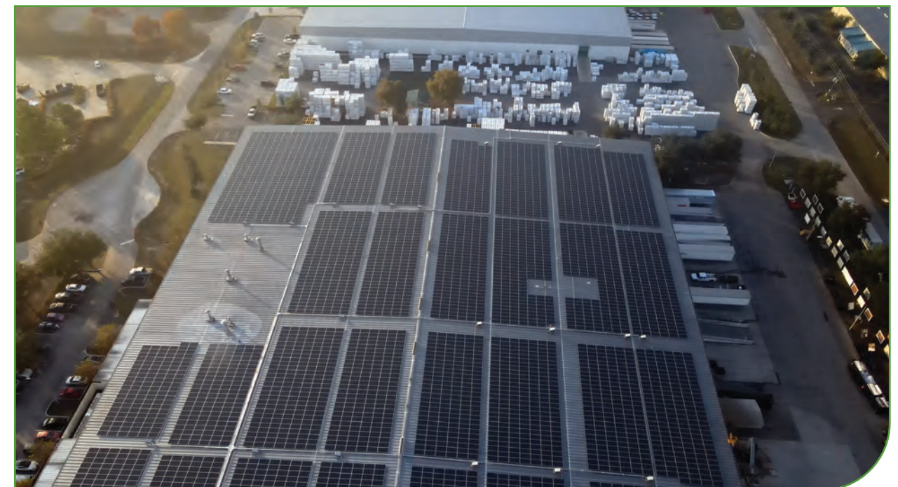
Rooftop solar array at plant in Brooksville, Florida
